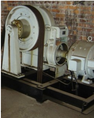
Geared Hoist Motor
