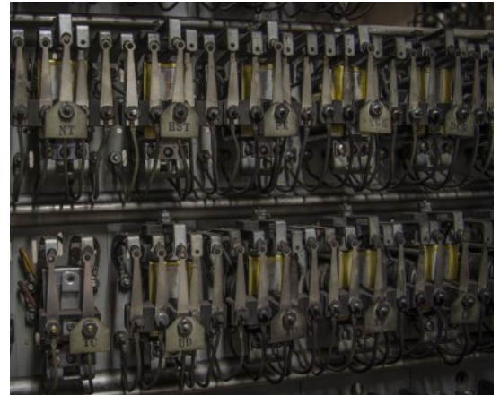
Old Style DC Relays
