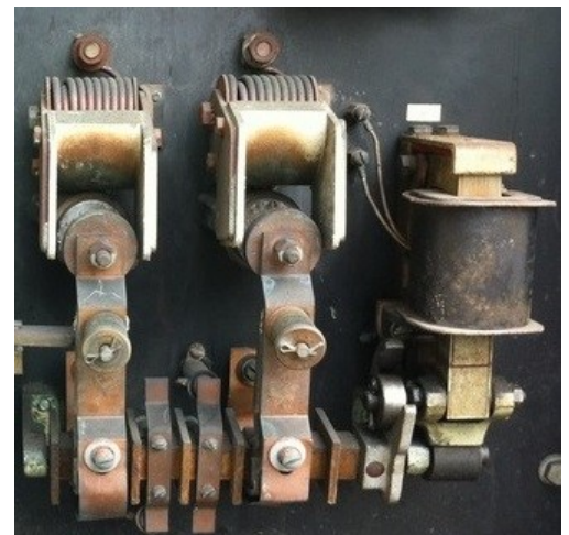
Older Style DC Contactor
